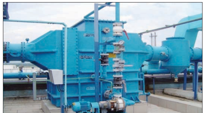
Horizontal scrubbing system.
