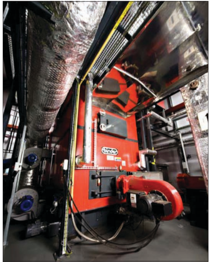
Biomass boiler fueled woodchip from sustainable forests.
