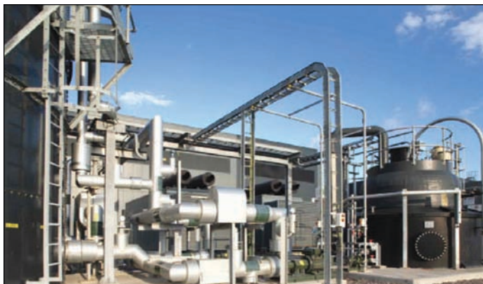
Centocor Biologics Ireland: Facility to capture rainwater from roofs within a grey water recovery system for future use in sanitary and ancillary process applications.
